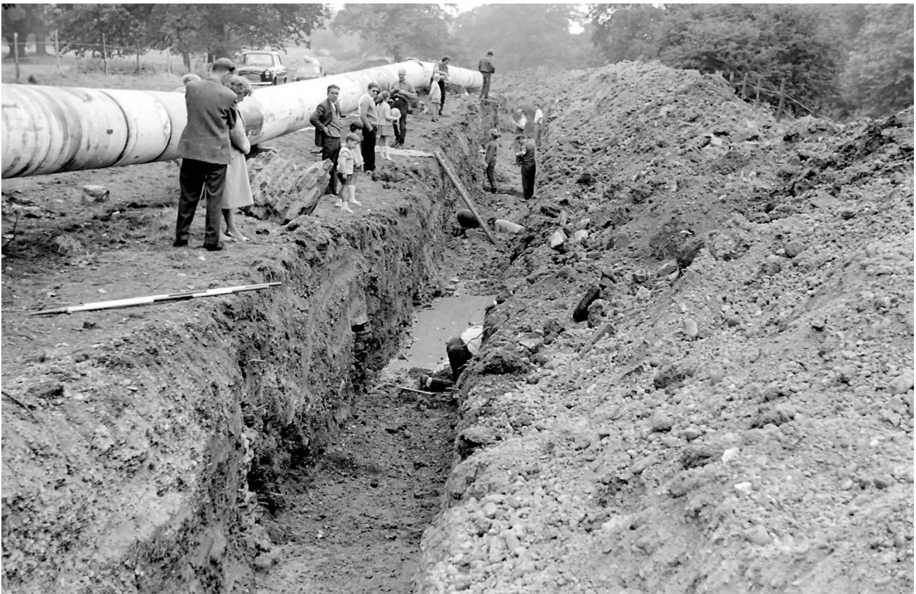
Pl. 1: The Gas Main Trench Looking West with [160] in the Foreground (Left Section) and Drain [159] Opposite the Nearest Excavator. The Flooding is in the Area of Walls [157] and [158].
